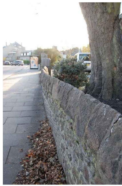
Boundary wall of The Fathers House (Former Rosemount Parish Church) adjacent to Caroline Place
