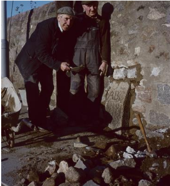
Fig.87 : Stone being reset into wall (photo courtesy of City Archives. c. ACC)
