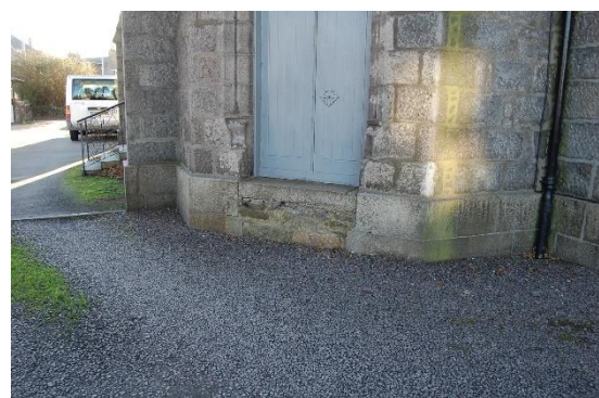
Fig. 20: Surface finishes and lack of steps to east side doors
