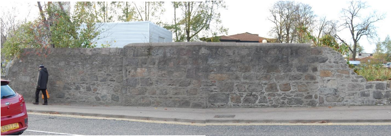
Fig. 76: Last section of Cornhill wall to left then former Asylum boundary wall going northwards, showing various phases of construction
