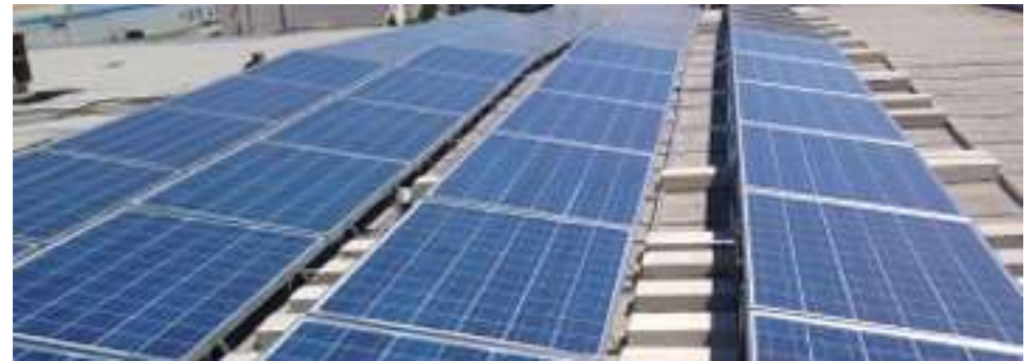
fig 71. plot one solar panels
