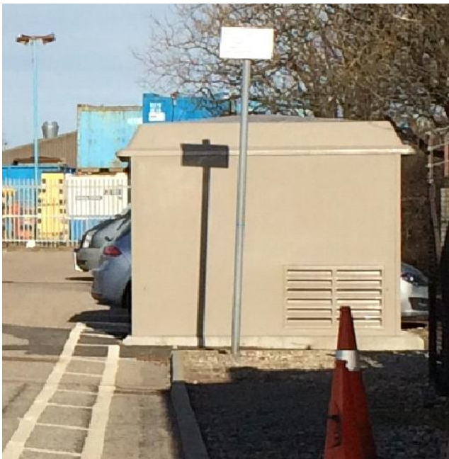
Figure 2.2 – Sub-Station in Dyce Station Car Park
