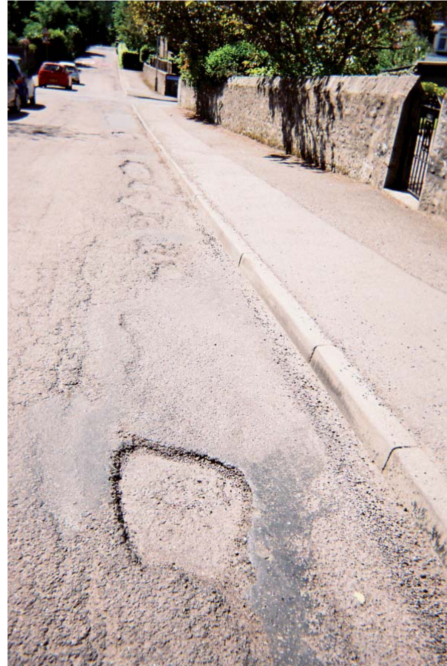
Potholes on Golf Road
