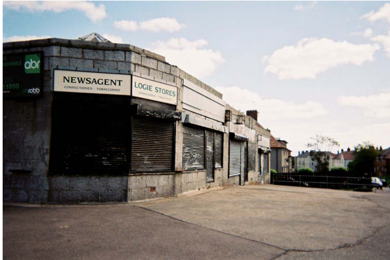
Derelict shops at Logie Place
