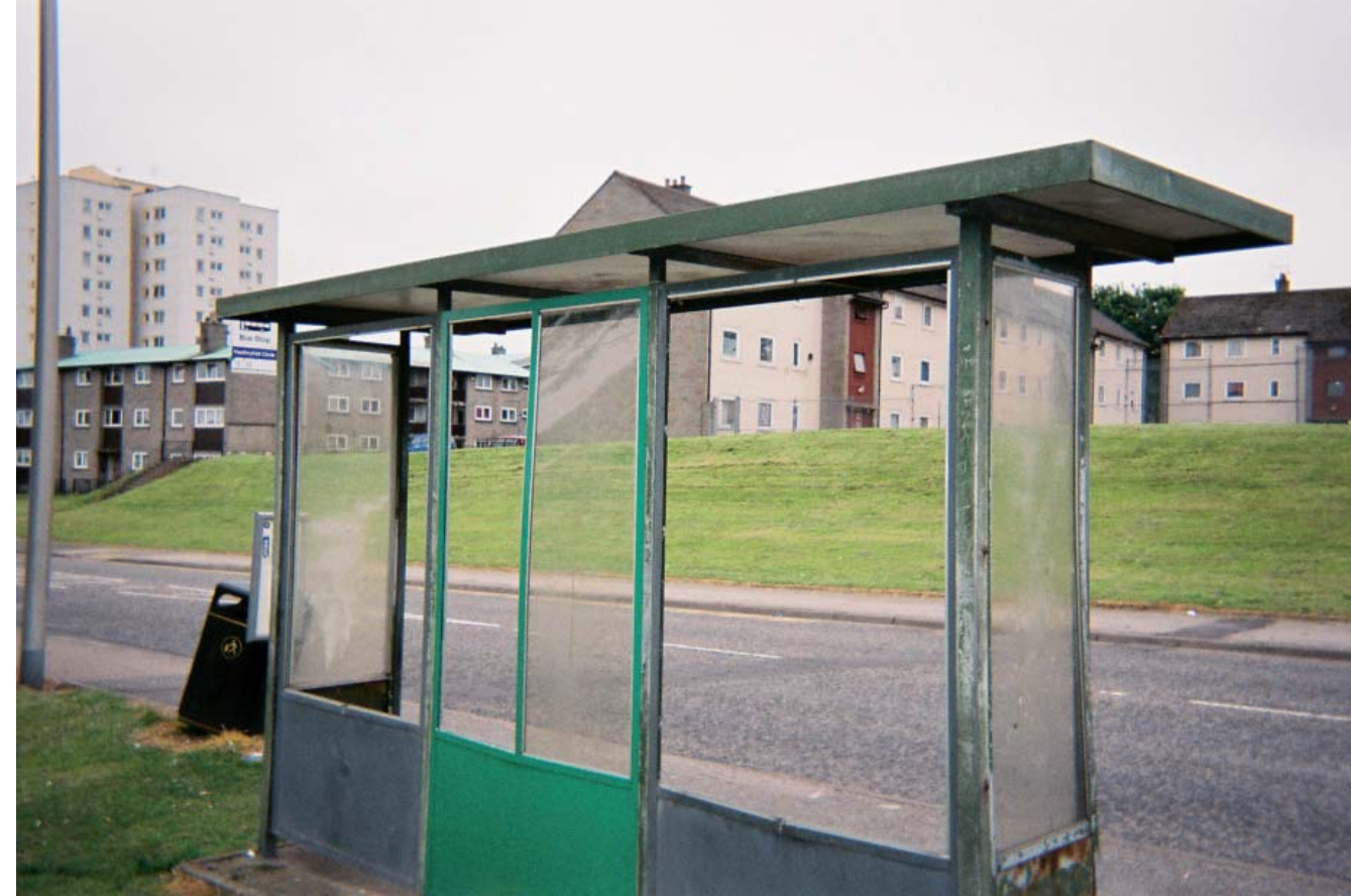
Bus shelter needs replaced
