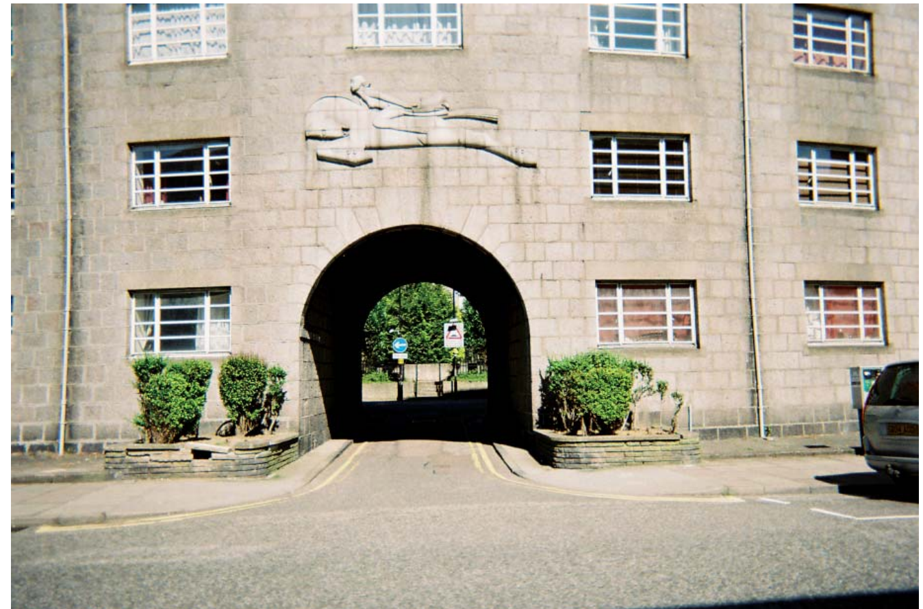
Poor upkeep of Council housing
