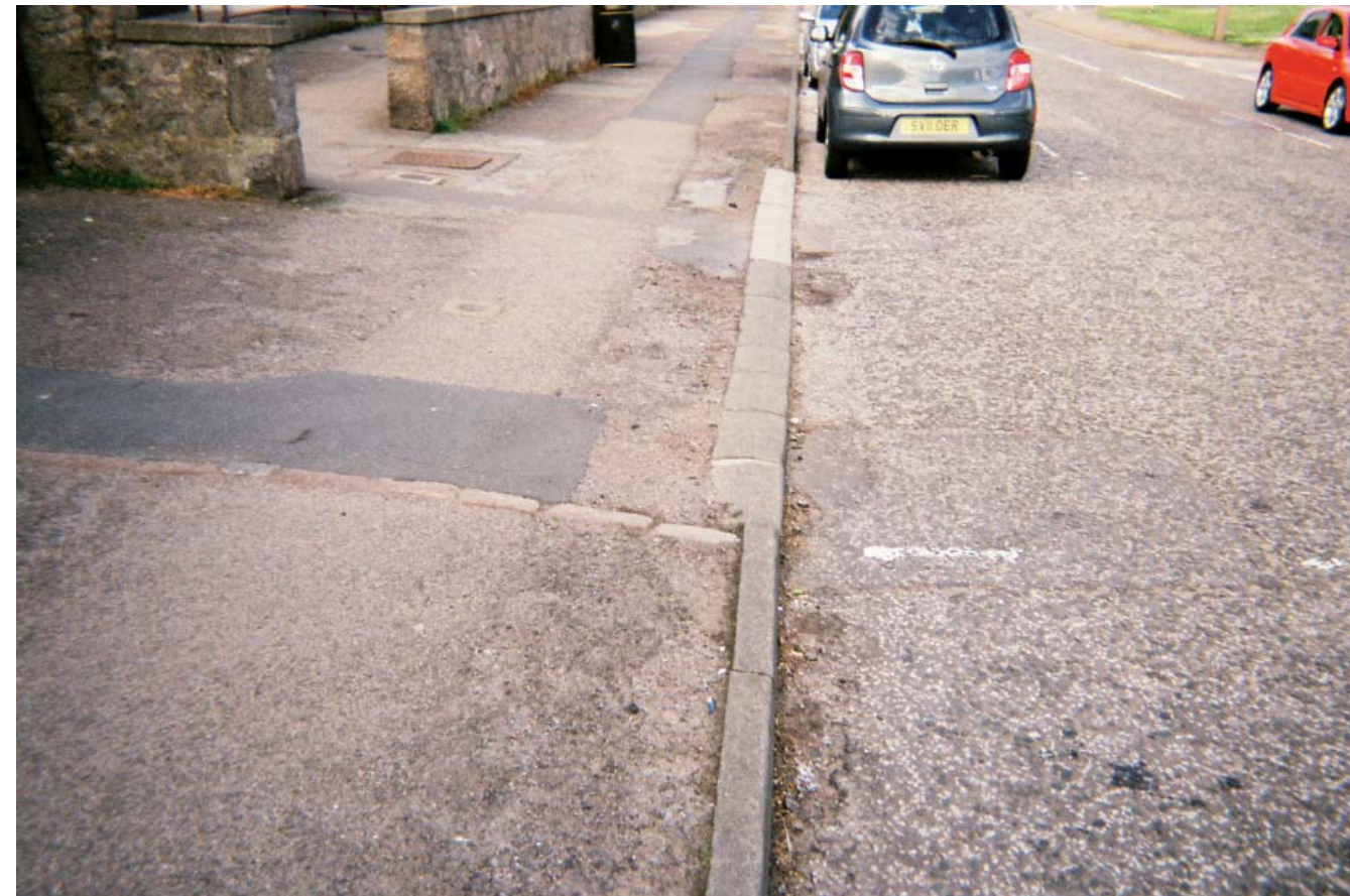
Poorly kept footpaths
