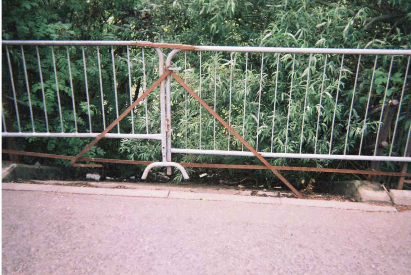
lack of access to jacobs ladder
