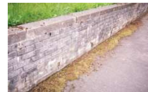
Poorly maintained pavements with moss
