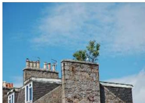
Poor maintenance of residential buildings
