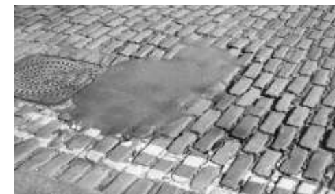
Inappropriate road repairs
