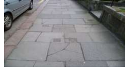
Broken paving slabs
