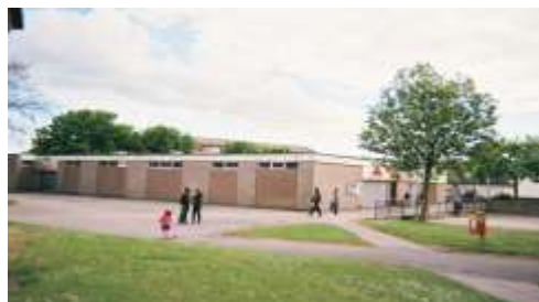
Local shops in a poor state of repair
