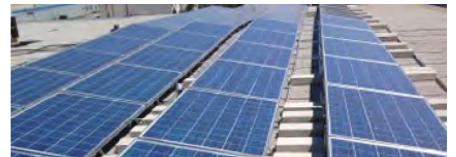
Figure 28: Plot One solar panels
