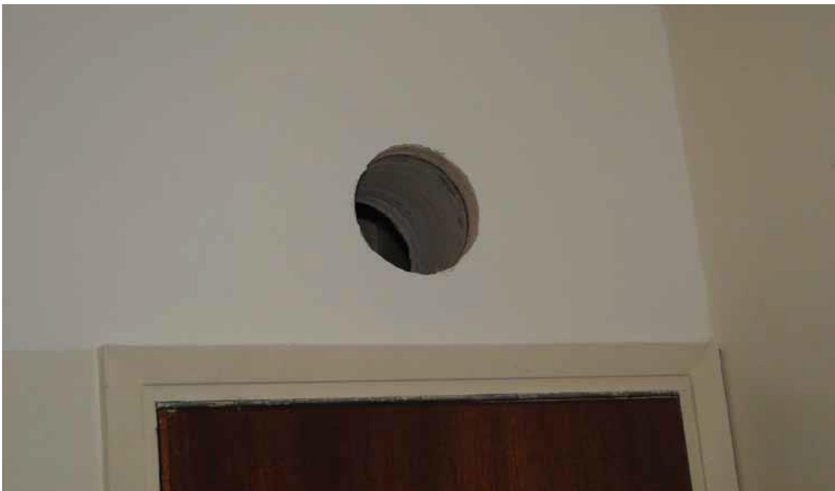
Figure 10 breach of fire-resisting enclosure
