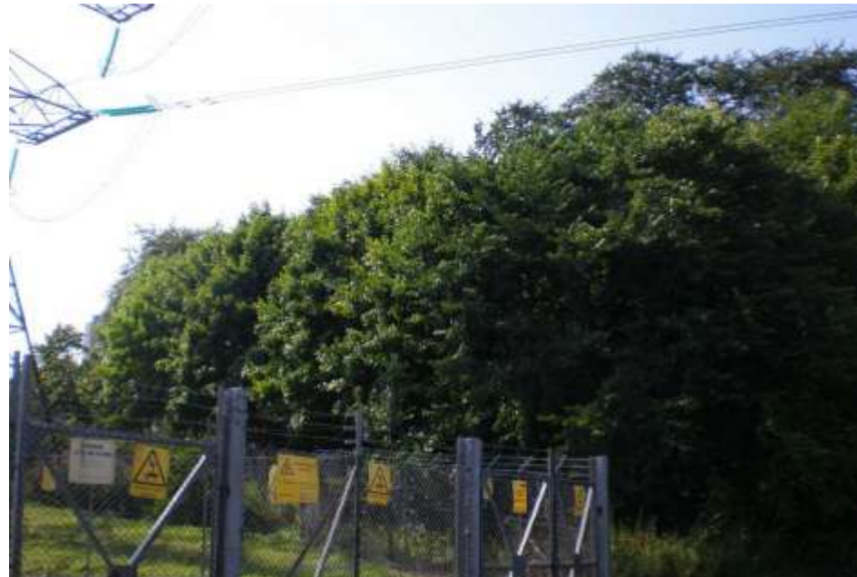
FIG 50: EXISTING SUB STATION COMPOUND
