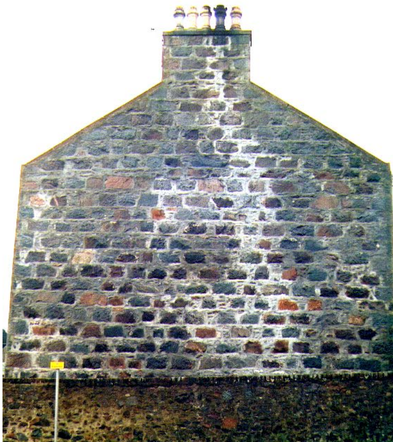
Plate 2.7 The dry patch on this gable appears to correspond to the position of fire places and flues.
