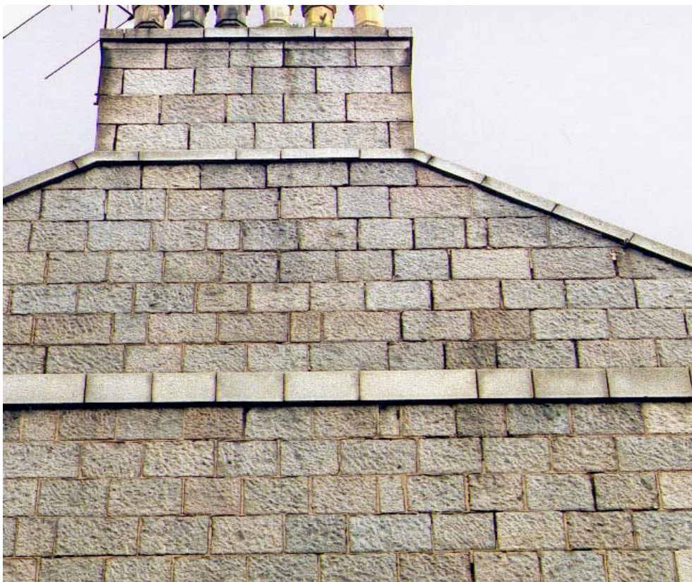
Plate 2.13 Most pointing mortar has been lost from both horizontal and vertical joints in the area of the chimney and on the right half of the wall.
