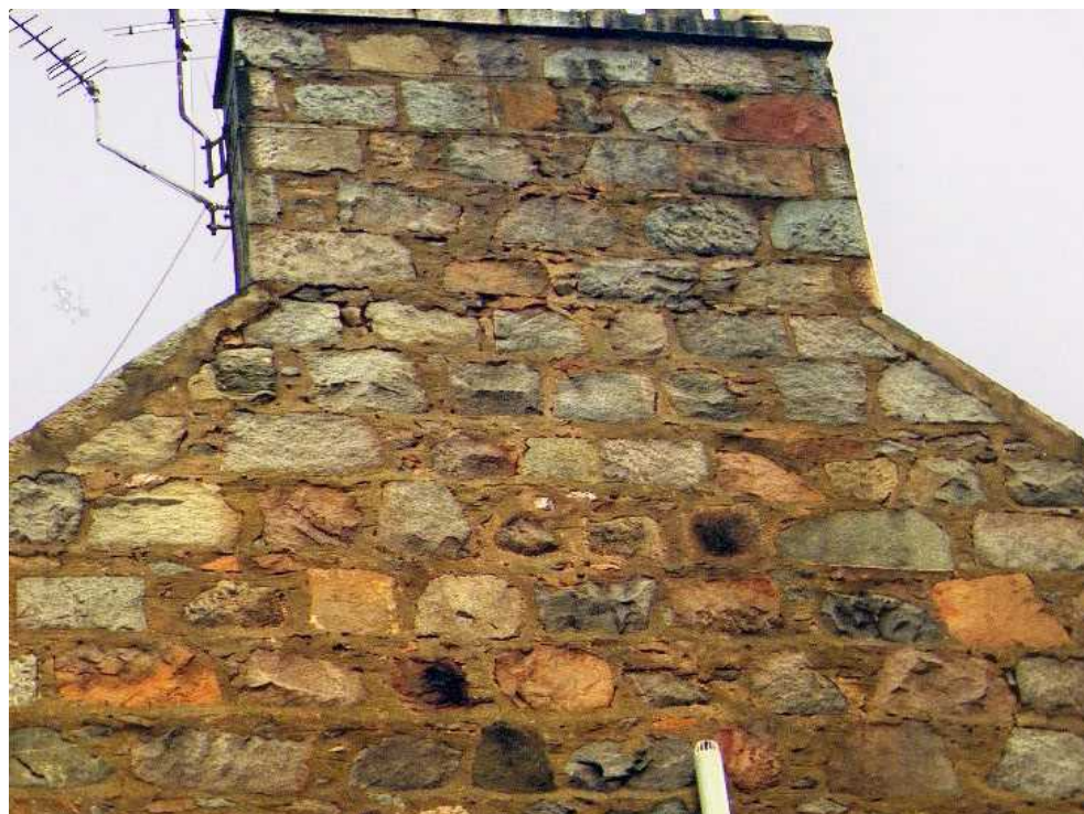
Plate 2.14 The pointing mortar on the upper area shown in this photograph is in very poor condition.
