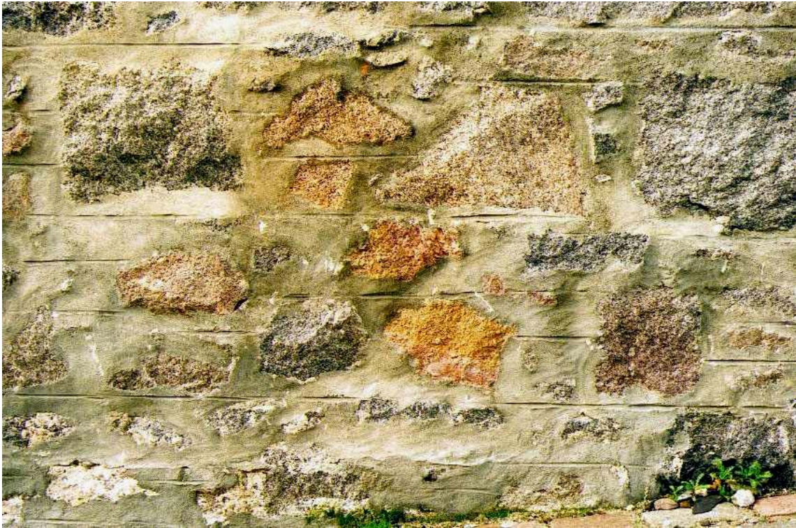
Plate 2.9 The pointing mortar dries more slowly than the granite since it is more porous and permeable and holds more moisture than the granite.
