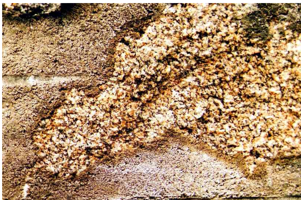
Plate 2.12 The darker features on this pointing mortar show the location of hairline cracks where more moisture has been taken up by the mortar.
