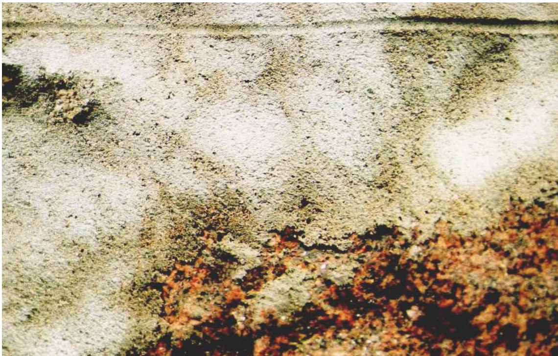
Plate 2.10 Where moisture can get easier access through cracks between mortar and stone, moisture is retained for longer. In this example, the mortar around the stone remains damp after the rest of the wall has dried.
