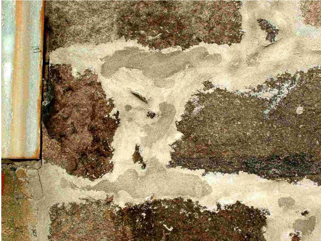
Plate 4.25 Two colours of mortar were visible on some areas of the gable (at its left end, as shown here) and on the front façade. The 'darker' coloured mortar was normally surrounded by 'lighter' coloured mortar.
