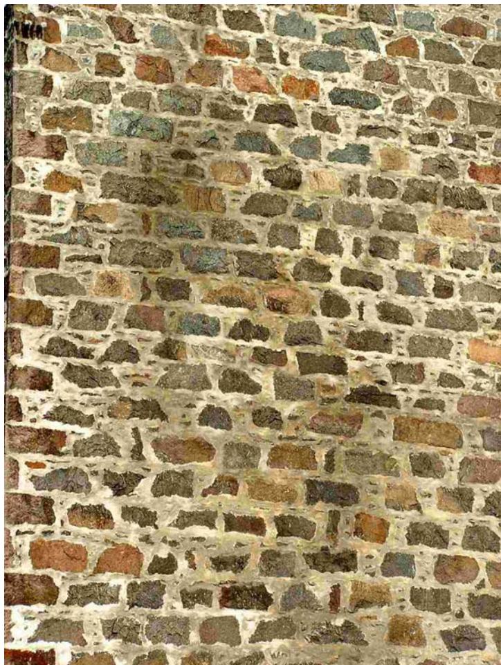
Plate 4.29 This close-up of the area to the upper left of Plate 4.28 (March 2003) shows darker, damp areas of pointing on the left and lower centre. There is an area with two differently coloured mortars (darker and lighter) in the upper right of the picture.
