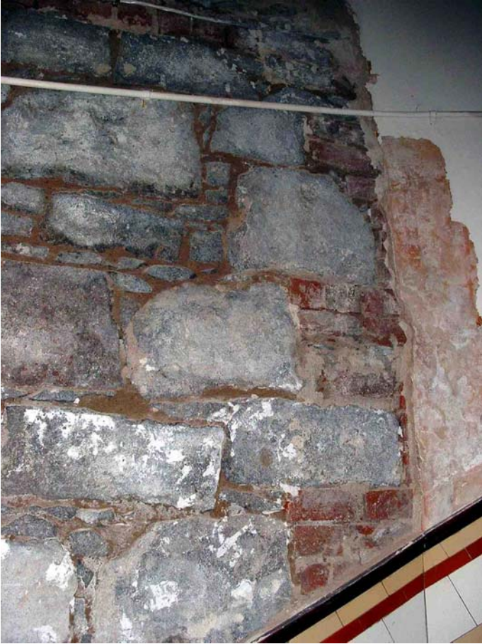
Plate 4.17 Plaster removed from area affected by dampness at first floor level (Feb 2003).
