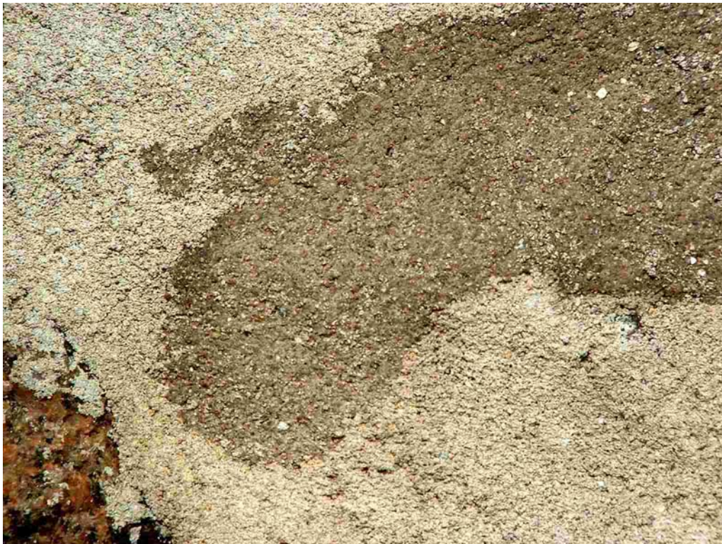
Plate 4.26 Close-up showing the 'darker' and 'lighter' coloured mortars at the left end of the gable. The darker colour is not caused solely by differences in degree of dampness although the 'darker' mortar here is damp and the 'lighter' mortar is dry (tested by electrical conductivity).
