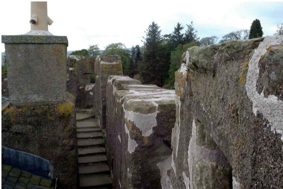
Plate 4.39 Roof of keep. The roof is well maintained and drainage is provided to minimise rainwater penetration into walls.
