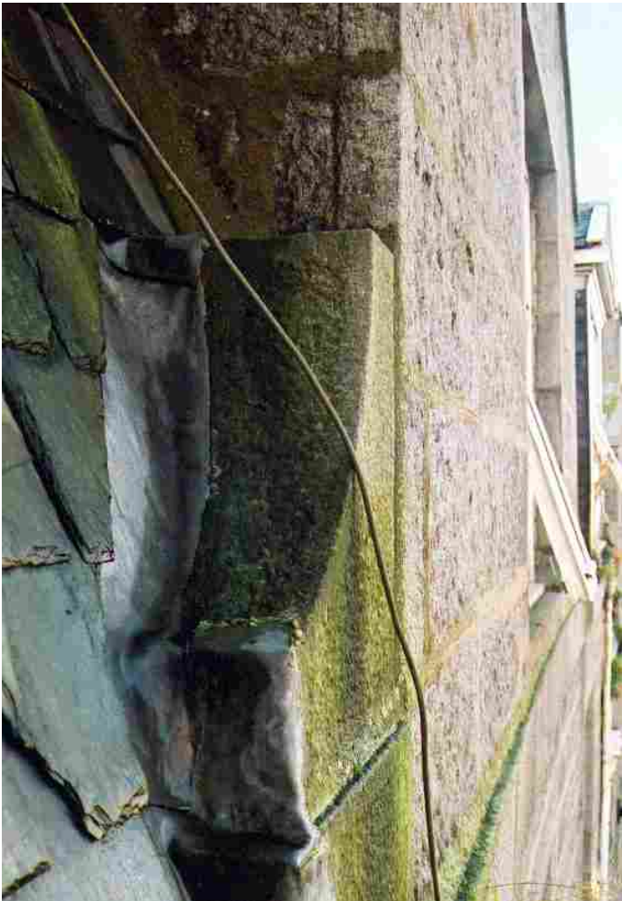
Plate 4.10 Detail at 3 rd floor level shows leadwork and green algae on stone indicating that some run-off comes from roof level.
