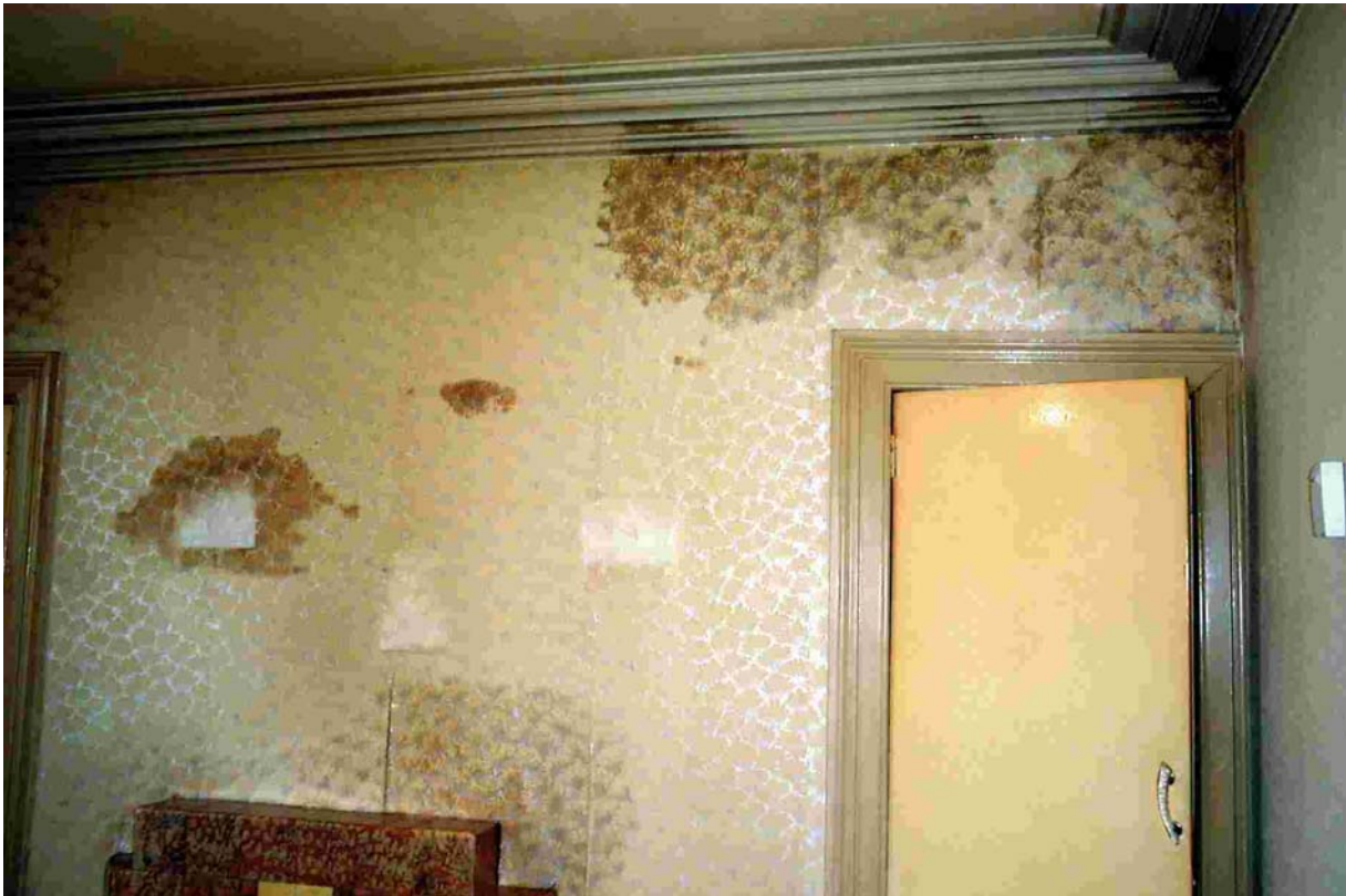
Plate 4.3 Dampness on internal gable wall.
