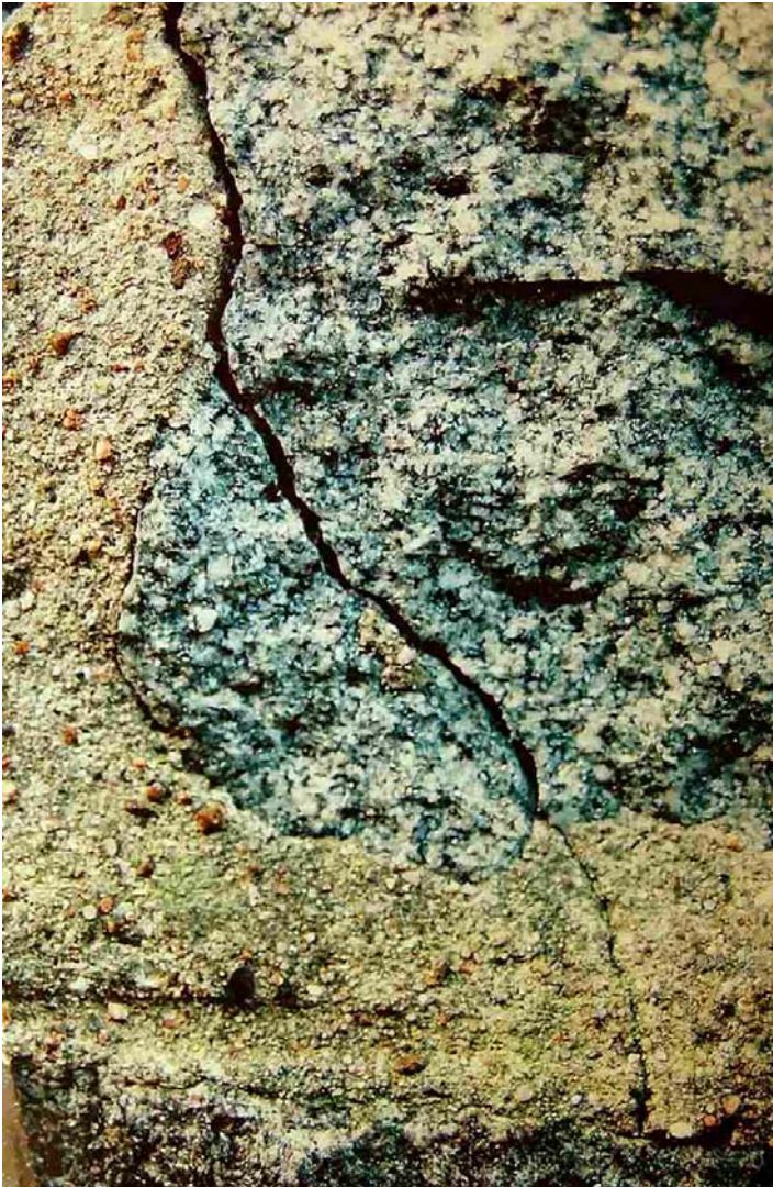
Plate 4.20 Cracked pointing and granite due to settlement.
