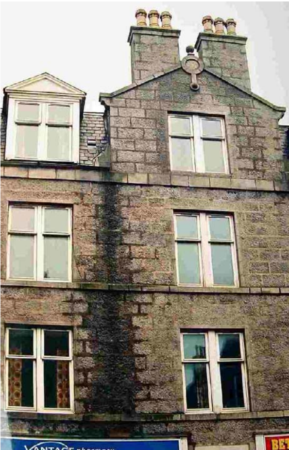
Plate 4.8 Front facade after a period of rain showing degree of wetting around area affected by rainwater run-off.
