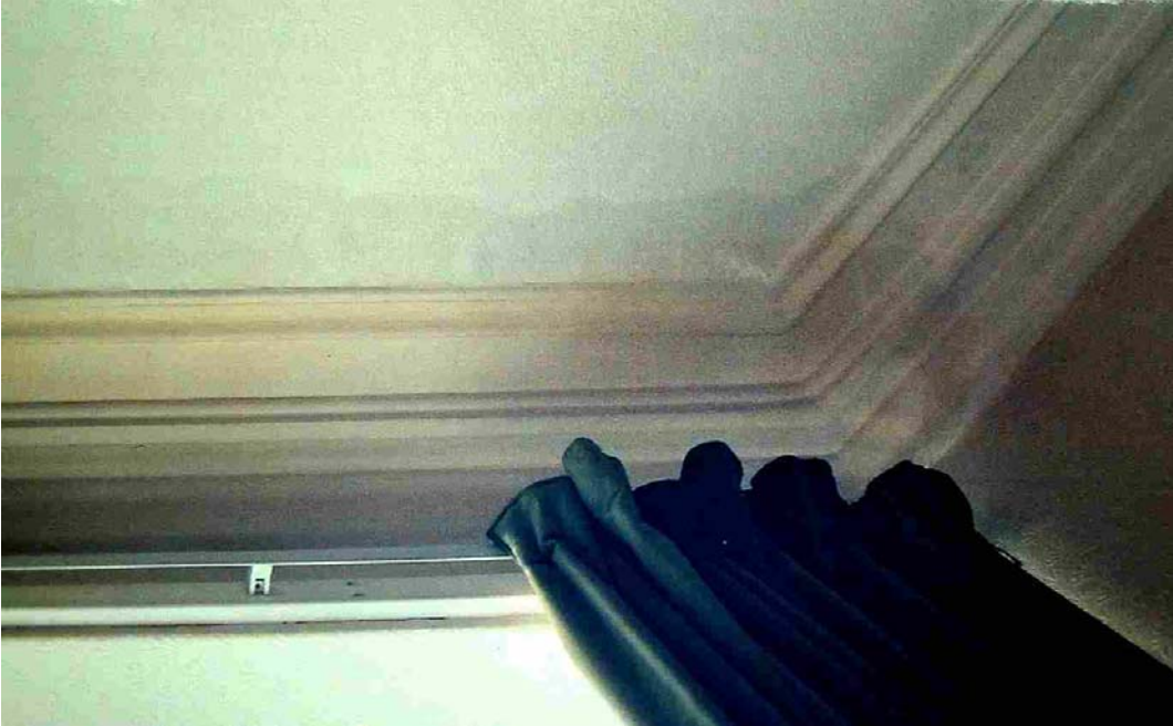
Plate 4.22 Damp patch above window.
