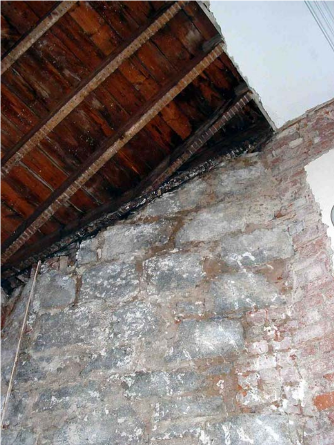
Plate 4.18 Plaster removed from area affected by dampness at upper level (Feb 2003). This revealed damp wood.
