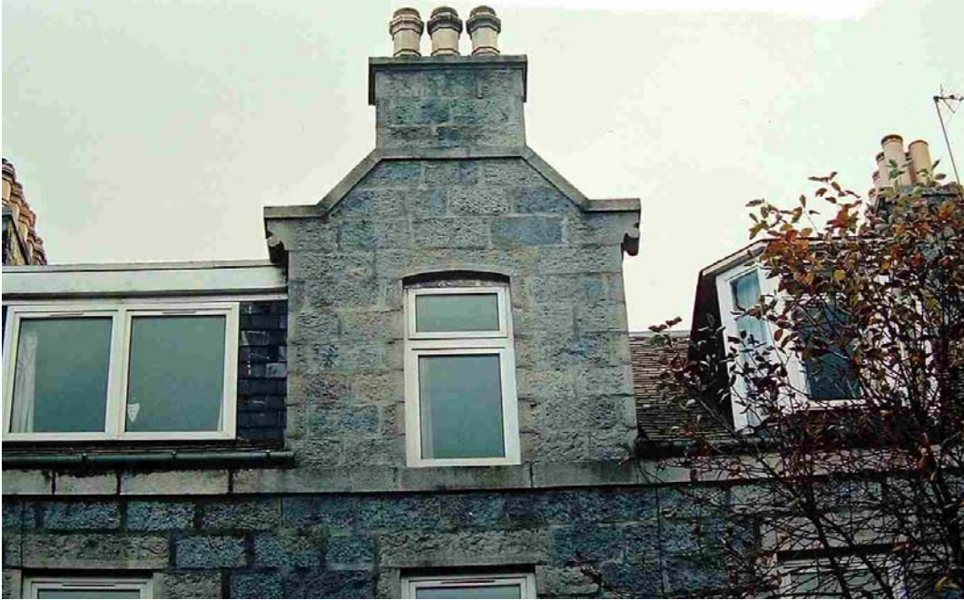
Plate 4.21 Case study five. Affected central bedroom on top floor with granite faced dormer.
