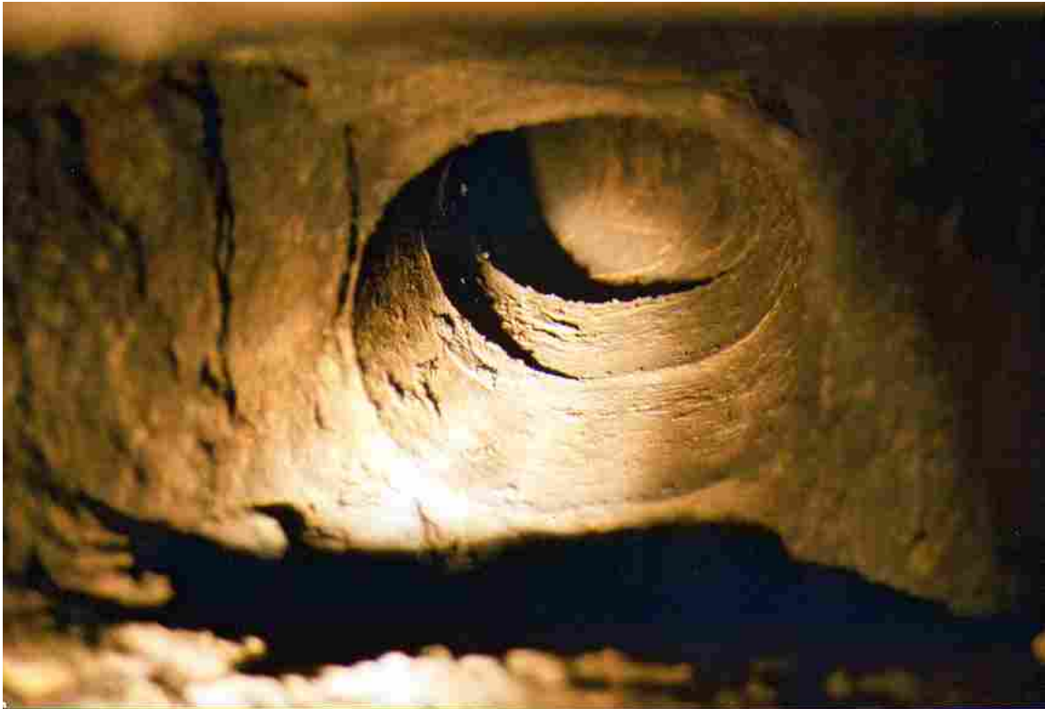
Plate 4.9 Flues are lined internally as can be seen in this view up a chimney.
