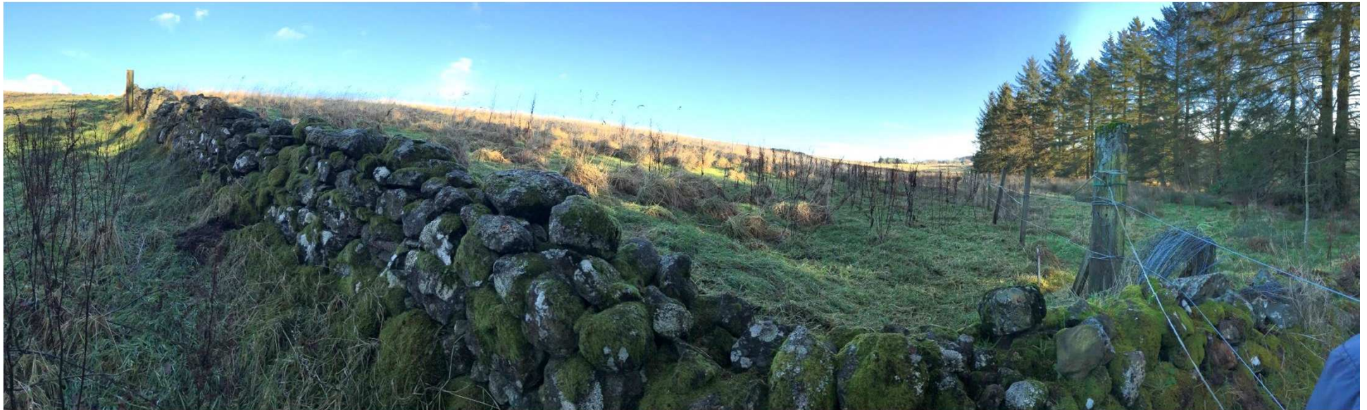
6. Dry stone wall field boundary at mid point of site looking north
